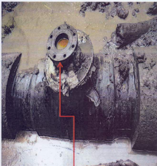
Fig D: 4" nipple/valve installed by Vandals
